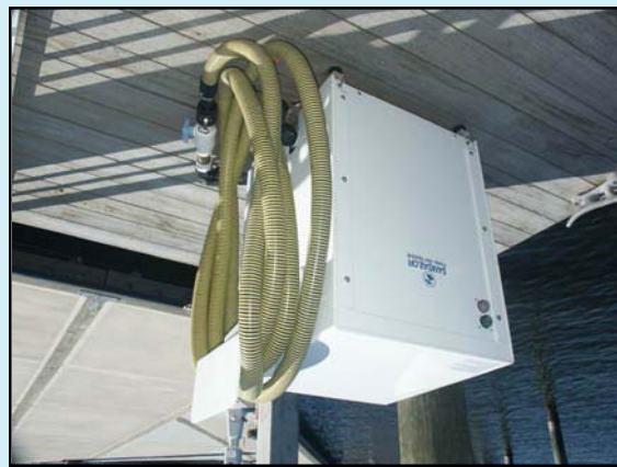
A marine toilet pump-out station.
